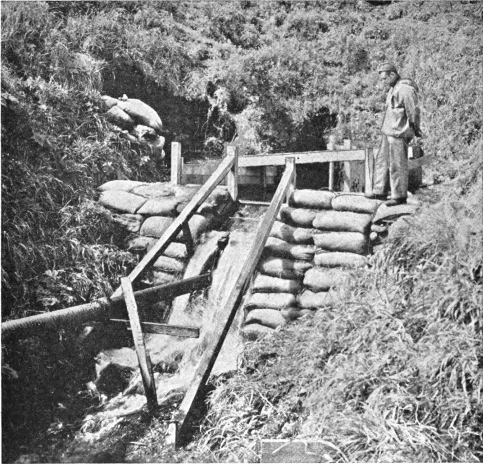
Figure 157. Water supply from spring.
